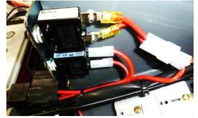
40A fuse with jumper shown installed
