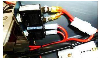
40A fuse with jumper shown installed
